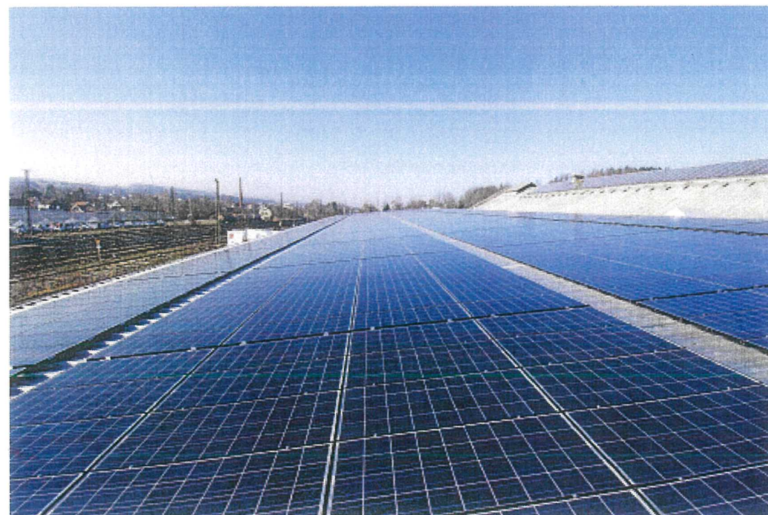
IMAGE EXAMPLE OF PHOTOVOLTAICS ON ROOF
